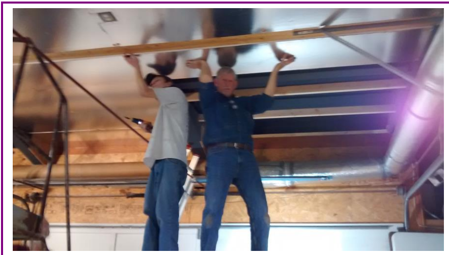
At left: Paul Jencka and Jake McClelland installing panels carefully around the area of the 16' garage door that connects the hangar to the meeting room.
